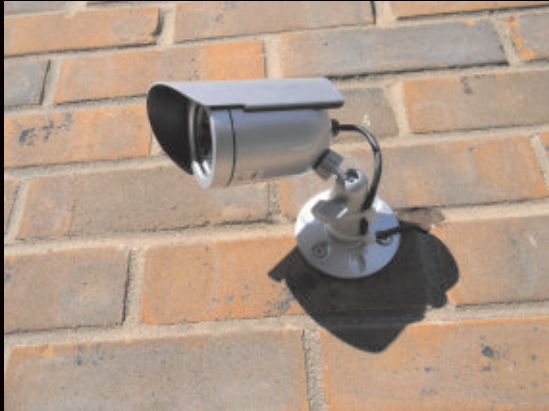
CCTV SECURITY CAMERAS
